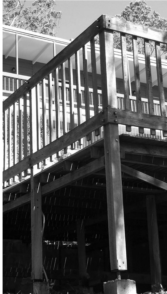
Additions and extensions need to meet construction requirements associated with the main building
