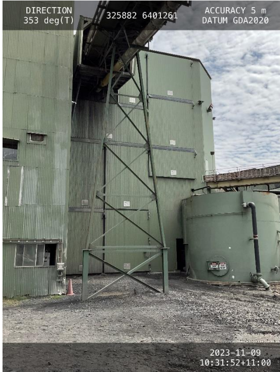
Plate 15: RCS Sound Cladding on CHPP.
