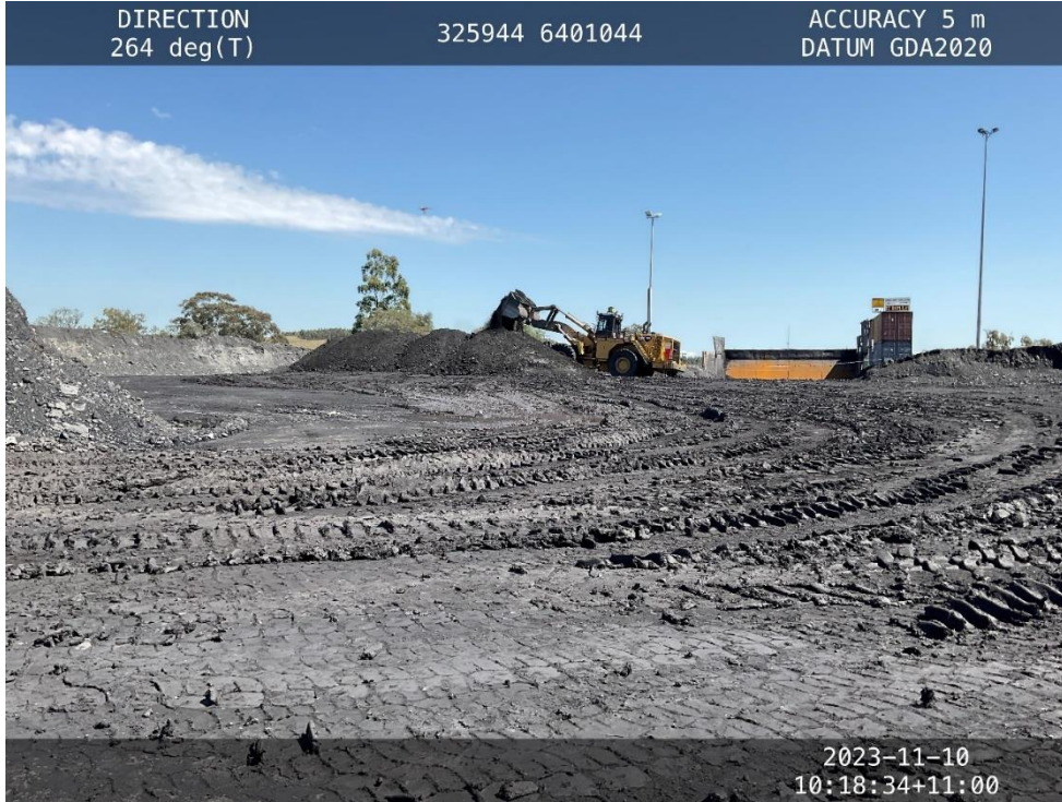
Plate 25: RCS ROM Pad.
