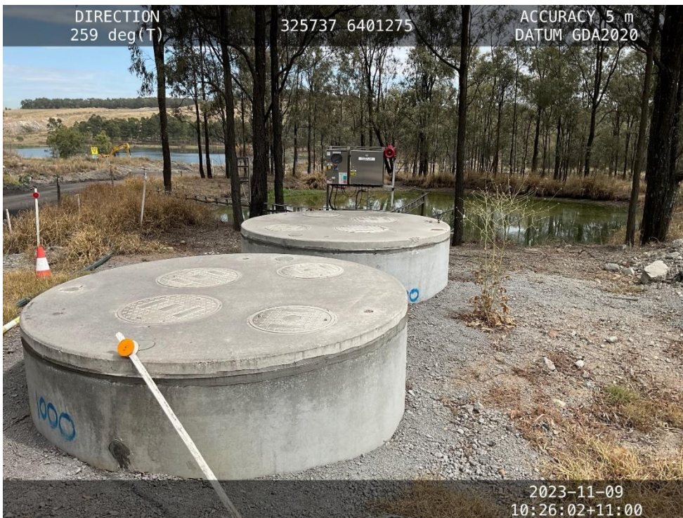
Plate 13: RCS Sewage Treatment Plant and Effluent Dam.
