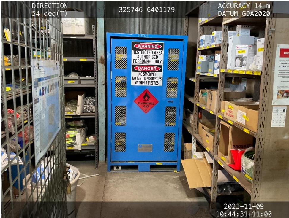
Plate 6: RCS Main Store Flammable Gas Storage.
